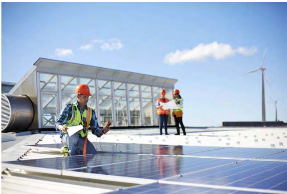
5G could allow for more efficient transmission and management of energy.
